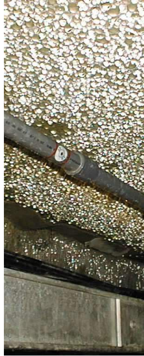
High humidity (cable tunnel)
